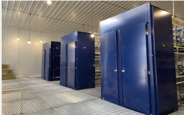
Automatic manure cleaning system
